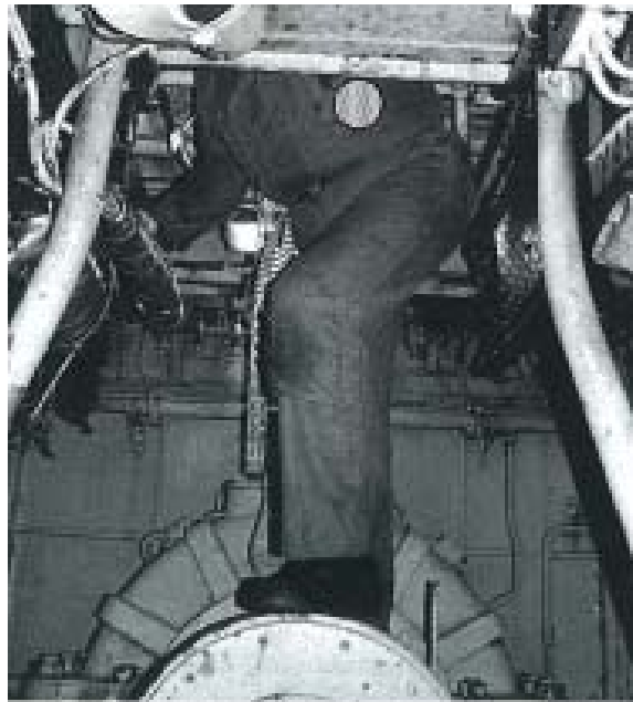
Fig. 3.16.1 Poor installed location of valve
