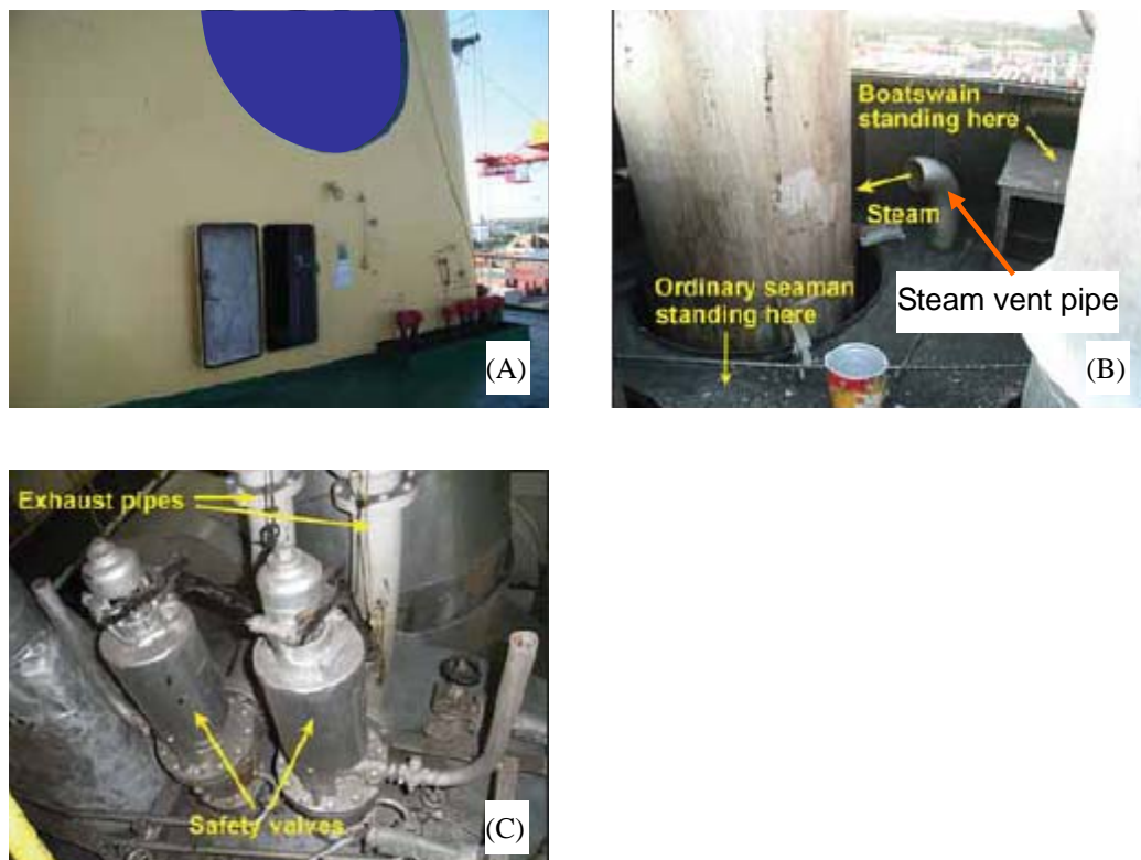
Fig. 3.3.1 Funnel, platform in funnel and boiler safety valves
