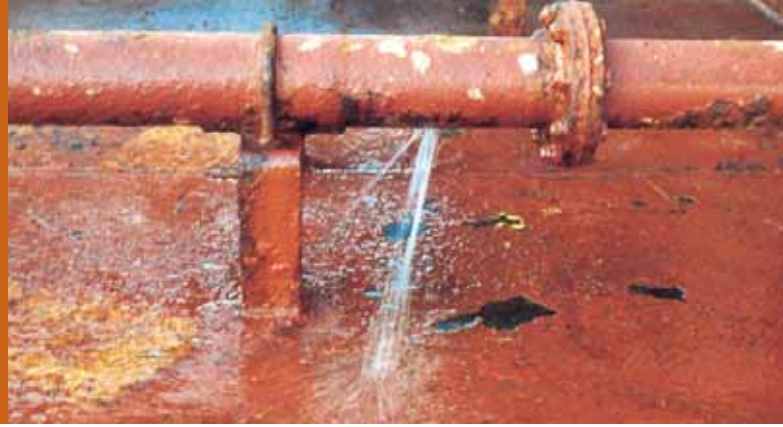
Image: Leaking fire main
