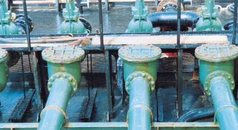
Image: Manifolds, filters and valves
