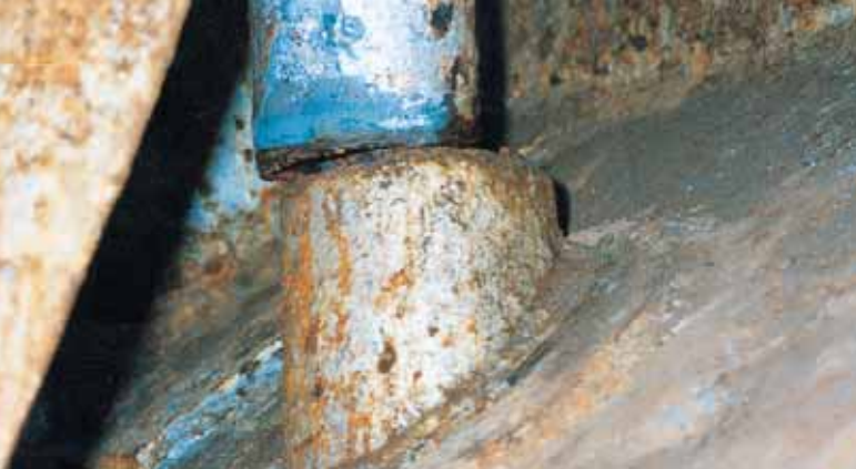
Image: Misaligned air ventilation pipe
