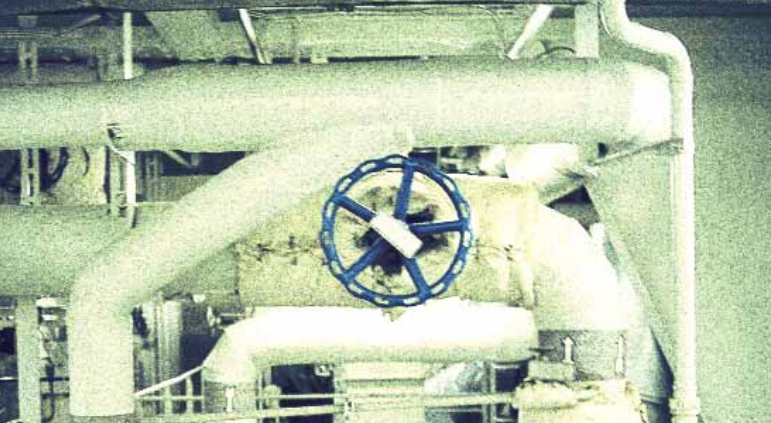
Image: Steam pipes
