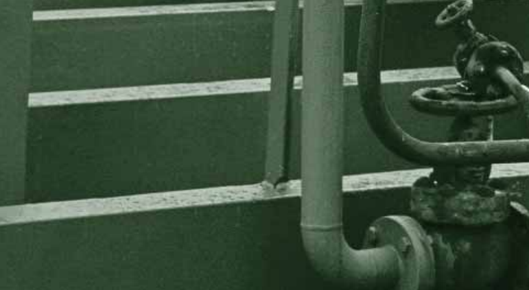
Image: Deck piping
