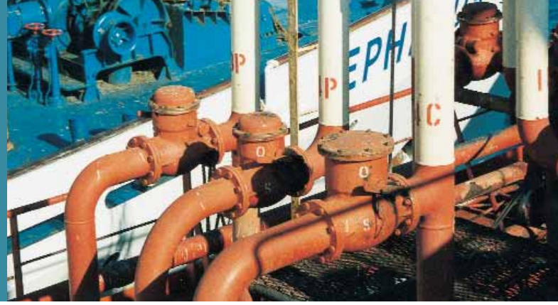
Image: Ventilation pipes
