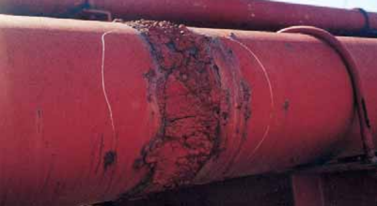
Image: Pipe corrosion
