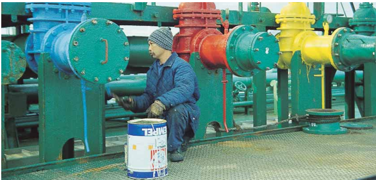
Image: Colour-coding cargo pipes
