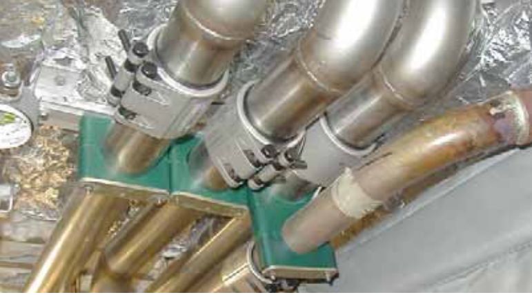
Image: Pipes with grip-type joints
