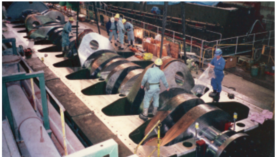
Fig. 17 The two-part crankshaft being installed in the bed-plate of the first 11RTA96C [7797-3030]
